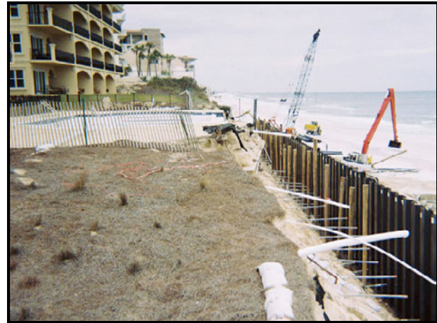
Protection of construction site using sheet-pile barrier and jute fiber mat (Source: Foundation Technologies, 2006)
