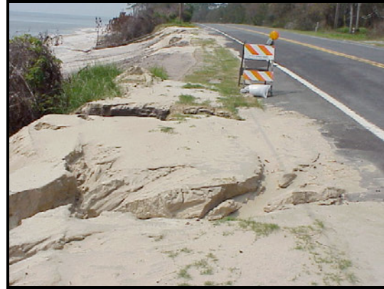
Sheet and gully erosion along shoulder, August 2005
