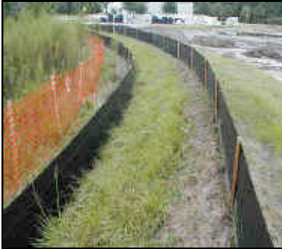
SRB prior to placement of mulch barrier (Source: Florida Dept. of Envr. Protection, 1988)
