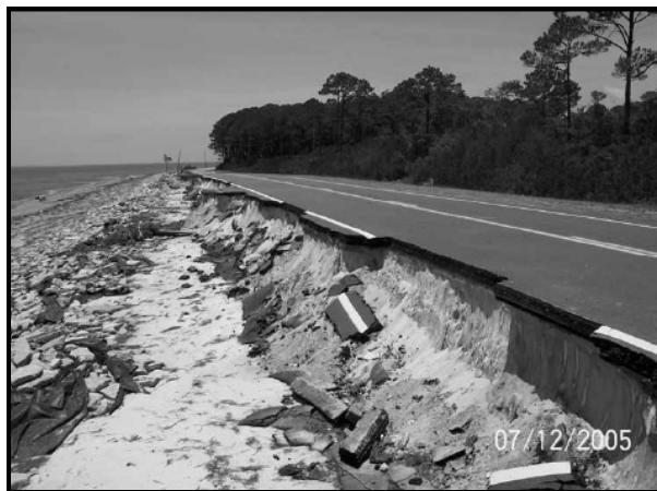
Front slope and shoulder damage on highway, July 12, 2005
