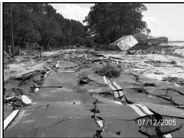
Full roadway damage on a portion of highway, July 12, 2005
