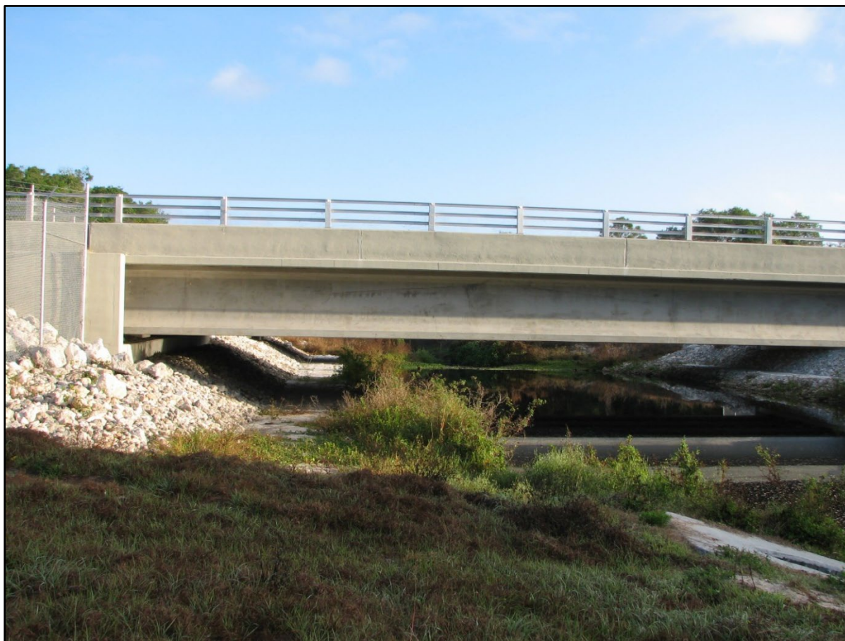
Figure 17 – 1 Bridge with Shelves for Wildlife
