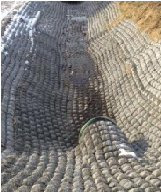
Flexamat or reticulated concrete channel
